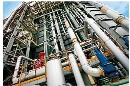
Pinjarra cogeneration plant
