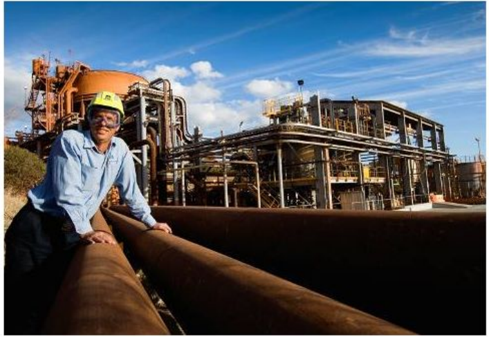
Carbon capture plant, Kwinana, Western Australia
